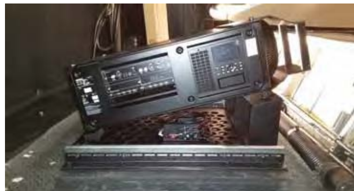
Projector 1 in the Griffith Observatory Samuel Oschin planetarium cove, installed September 23 rd . Video cables, mask and lens were not yet attached. Photo courtesy Griffith Observatory.
